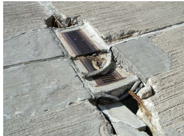
Deteriorated Joint and Drain
